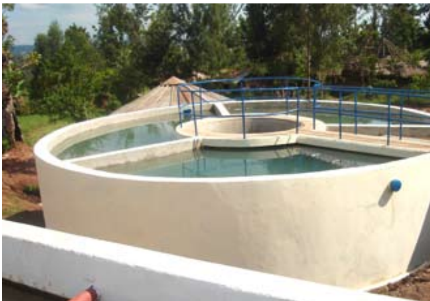
Angurai water supply
